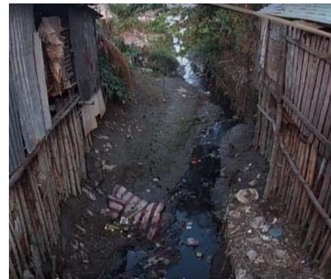
Linkage of City drain with Rupsha river
